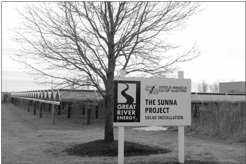
A "community garden" solar facility is located near the Steele-Waseca Cooperative Electric facility in Owatonna. The field of solar panels is about one-third acre in size, and provides electricity for SWCE members.
