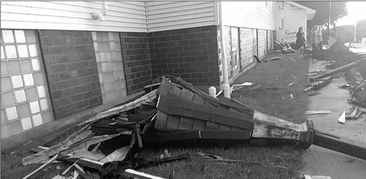
The bell tower and steeple of LeSueur River Lutheran Church, located northeast of New Richland, were broken loose by a tornado in June of 2020 and dropped to the ground nearby. The remainder of the building was relatively untouched. The church was originally built in 1875.
